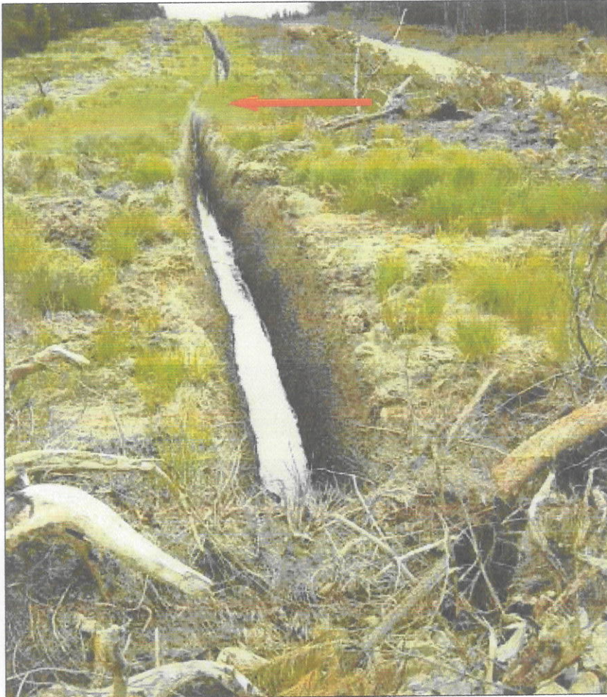
Plate 10.2: A ditch that runs ENE from T53 alongside a floating road across the northern slope of the mountain has obviously bowed and slumped downslope where it crosses deep peat. (It is assumed it originally ran straight.)
